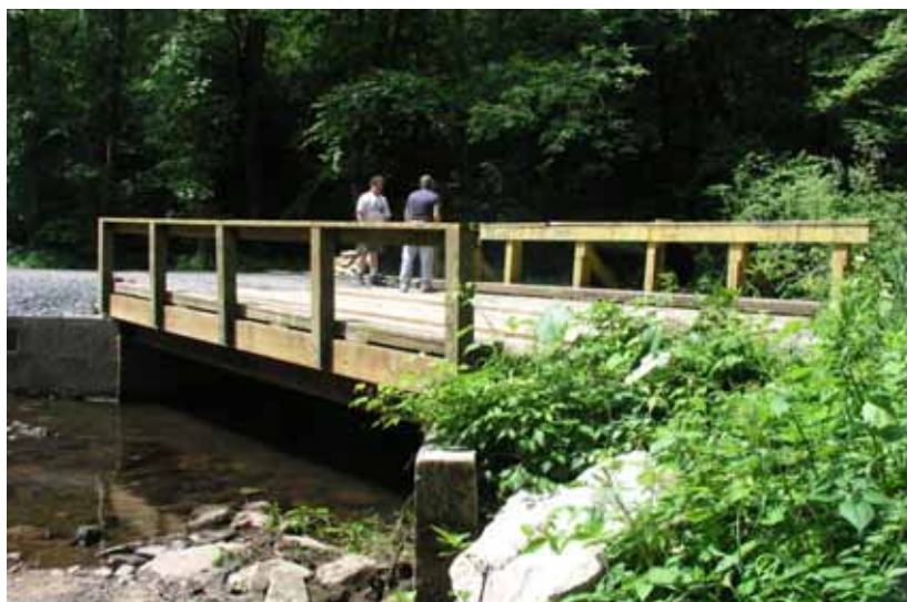
Reparation of the bridge over Stony Creek at Cold Springs. The original bridge was damaged by Hurricane Ivan rain storms.
